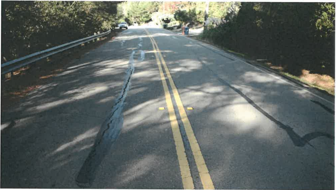
Rheem Blvd PCI 70
