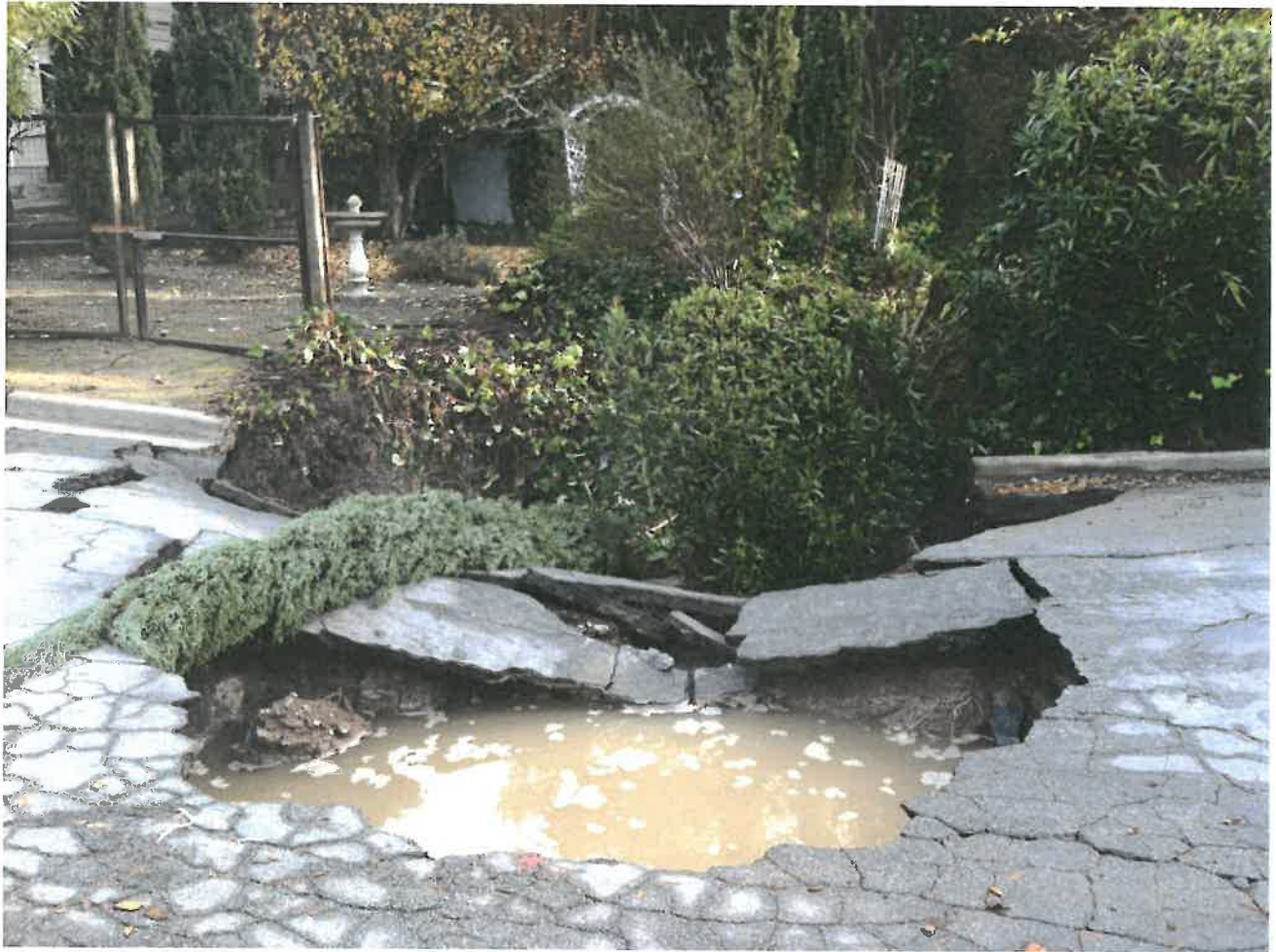
Storm Drain Failure on Tarabrook Drive at Evergreen Drive
