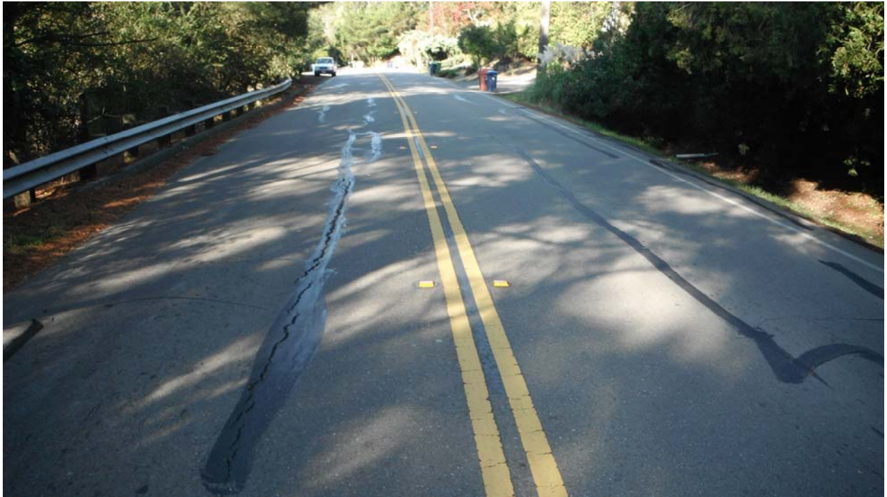
Rheem Blvd PCI 70
